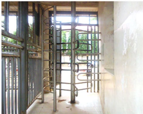
Plate IV: Turnstile access control mechanism at Federal Capital Development Authority Complex, Abuja. Photo credit: Samuel Ebong
